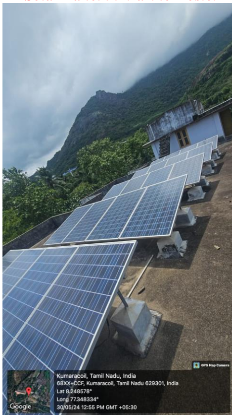
Solar Panel in Marine Hostel
