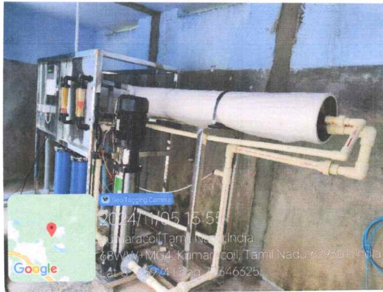
RO Plant in Gent's Hostel
